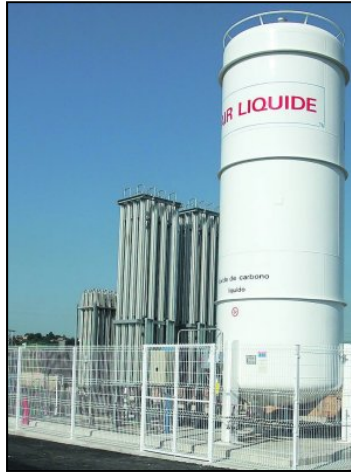
Figure 11-2. CO 2 storage tanks in “La Presa”. Source: EMV-Levante, 2010.
